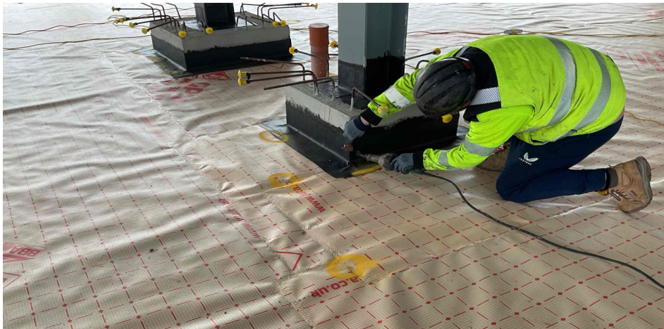
Fig. 11: Work being progressed, with areas that require attention/ remedial repairs clearly highlighted for action. Image credit: Nairn Academy, Balfour Beatty.
