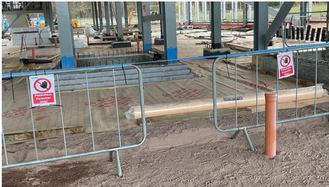
Fig. 21: Areas clearly delineated, with signage highlighting only trained personnel shall have access. Image credit: Nairn Academy, Balfour Beatty.
