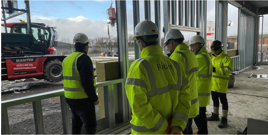
Fig. 3: Quality checking during the construction of Passivhaus project Paisley Grammar School. Image credit: Morrison Construction
